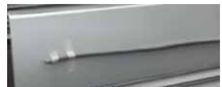
Backer rod installed on backside of metal panel to prevent oil canning
