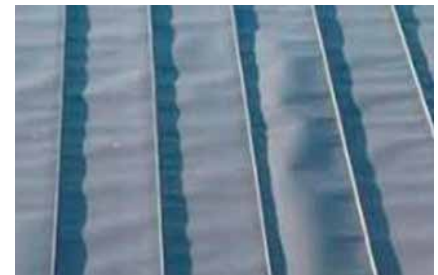
Oil canning on metal roof
